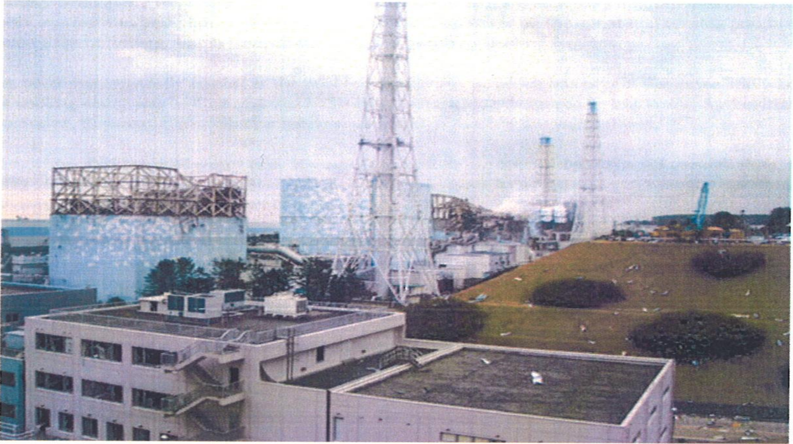
Damage is seen at the Fukushima Daiichi nuclear plant, and white smoke rises from reactor No. 3. The nuclear plant suffered heavy damage following explosions that occurred after last week's magnitude 9.0 earthquake off the coast of Japan. (EPA / TEPCO / March 16, 2011)
